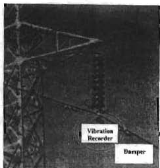
Fig. 1.a. Vibration recorder clamped to the wing (Two Mass-Dampers are clamped to the line).
