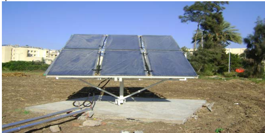
Fig. (2): Solar collector panel array, with a total surface area of 12.0 m 2 and mounted on a movable frame.
