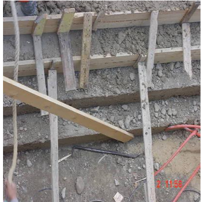
Fig. 21: No formwork removal for the previous casted layer
