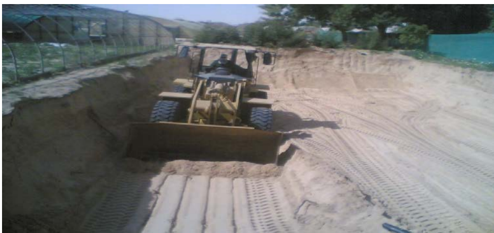
Picture (1): the depth of drilling into the study for the development of underground pipes
