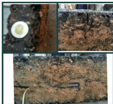
Figure 15. Cracks in AC Layer of the Control Section
